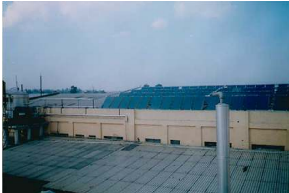
Solar water heating system at Leo Leather Industry, Jalandhar
